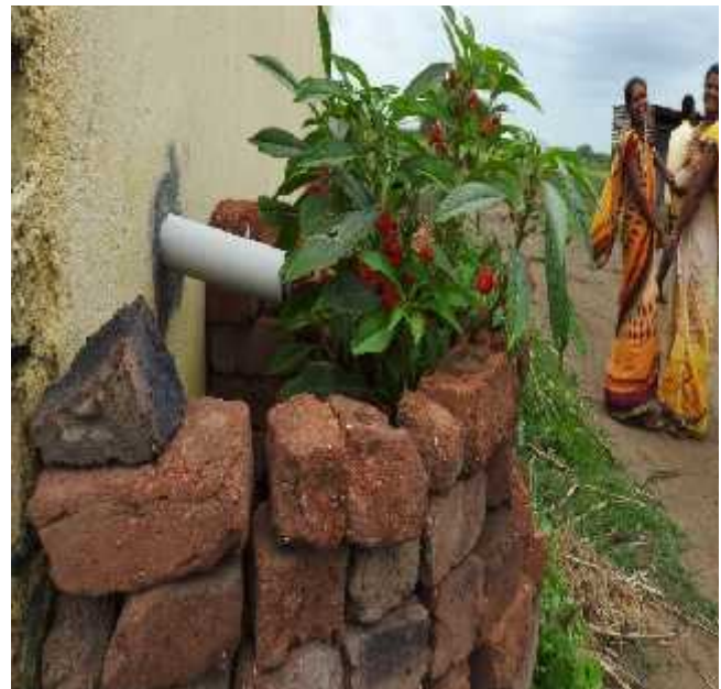
Simple pipe takes waste water from kitchen and provides water for small plants instead of being wasted
