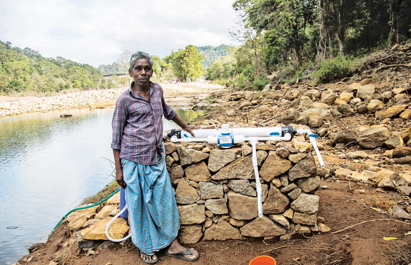
Madhavan, Community Leader of Peringalkuthu Kadar Colony mobilized community members to build a plinth for the water filter.
